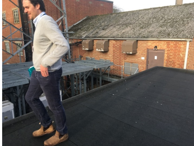
Lack of Edge Protection
