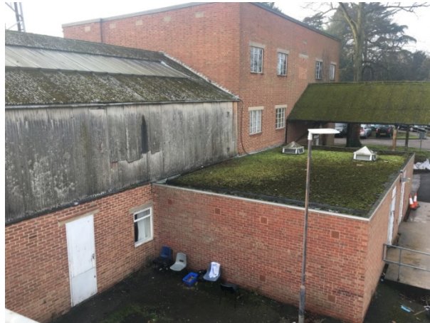
Asbestos Roof Panels to Supplies
