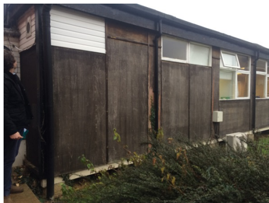
OPD Portacabin in Poor Repair
