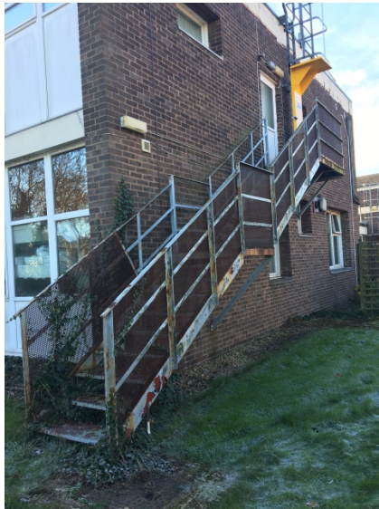
Unprotected External Fire Escape Stair
