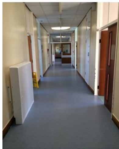
Fire doors requiring replacement
