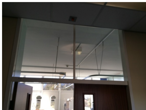
Integrity between door and overhead glass panel
